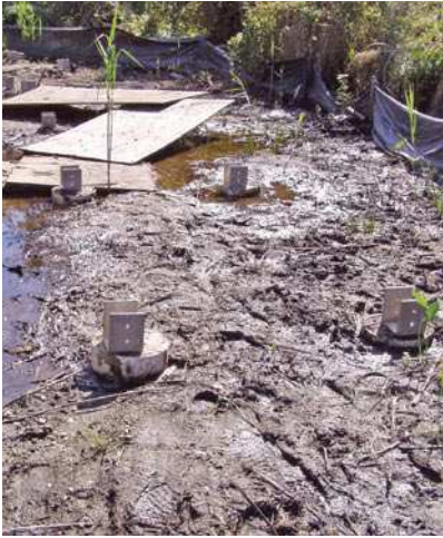
Failed foundation system
